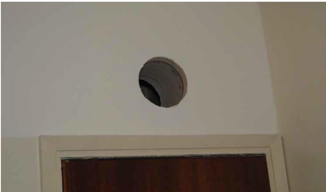
Figure 10 breach of fire-resisting enclosure
